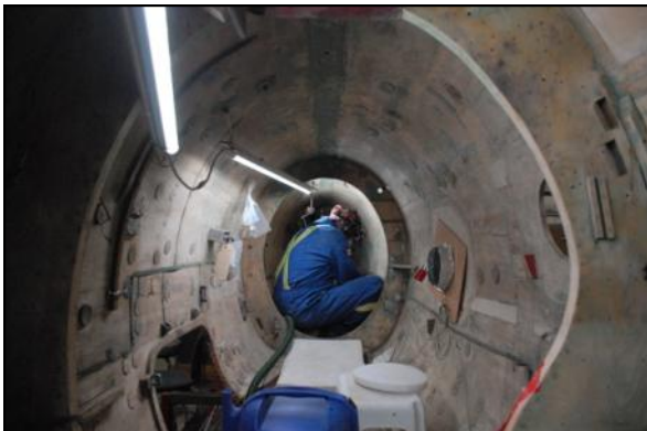
Another "inside job." A CMS volunteer works at a repair inside the fuselage.
