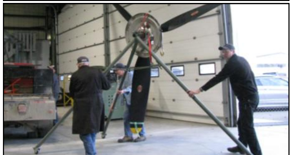
Carl Orde and Greg Morrison move the propeller into position for installation.
