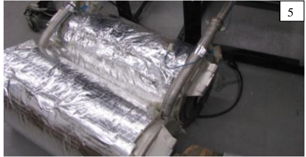
Two of the original heat exchangers.
